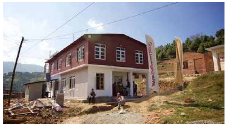
Before (above) and After (below) of the new clinic building in Bajra Barahi. Opened in October 2015
